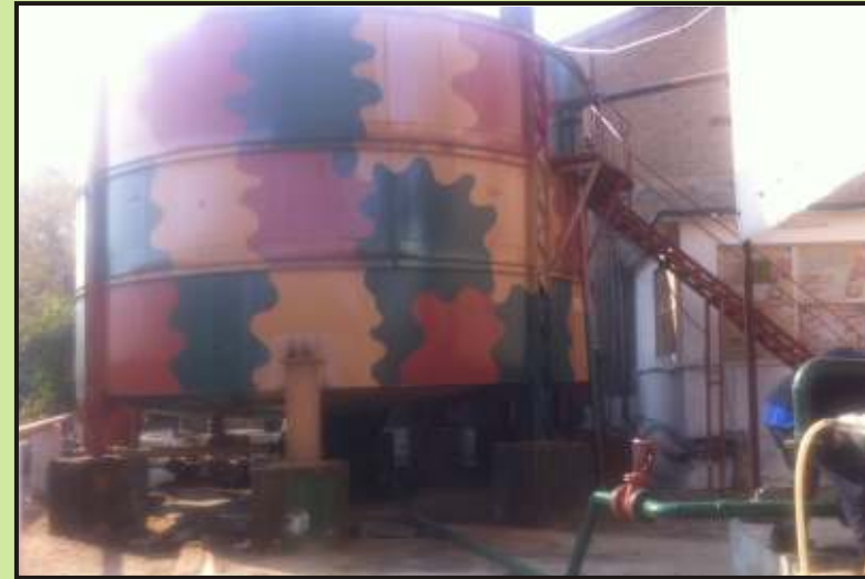
SECONDARY TREATMENT PLANT
