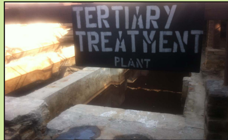
TERTIARY TREATMENT PLANT
