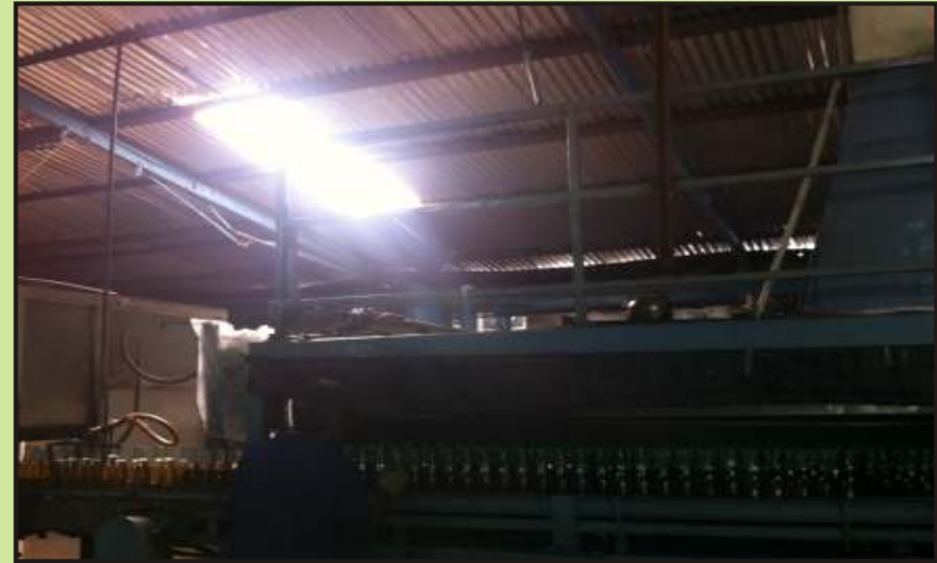
SKY SHEETS IN PRODUCTION HALL
