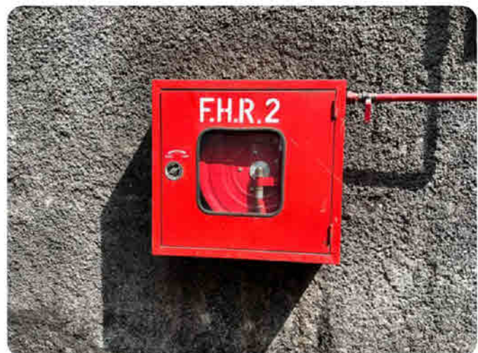
Upgraded Firefighting and Automatic Sprinkler Systems
